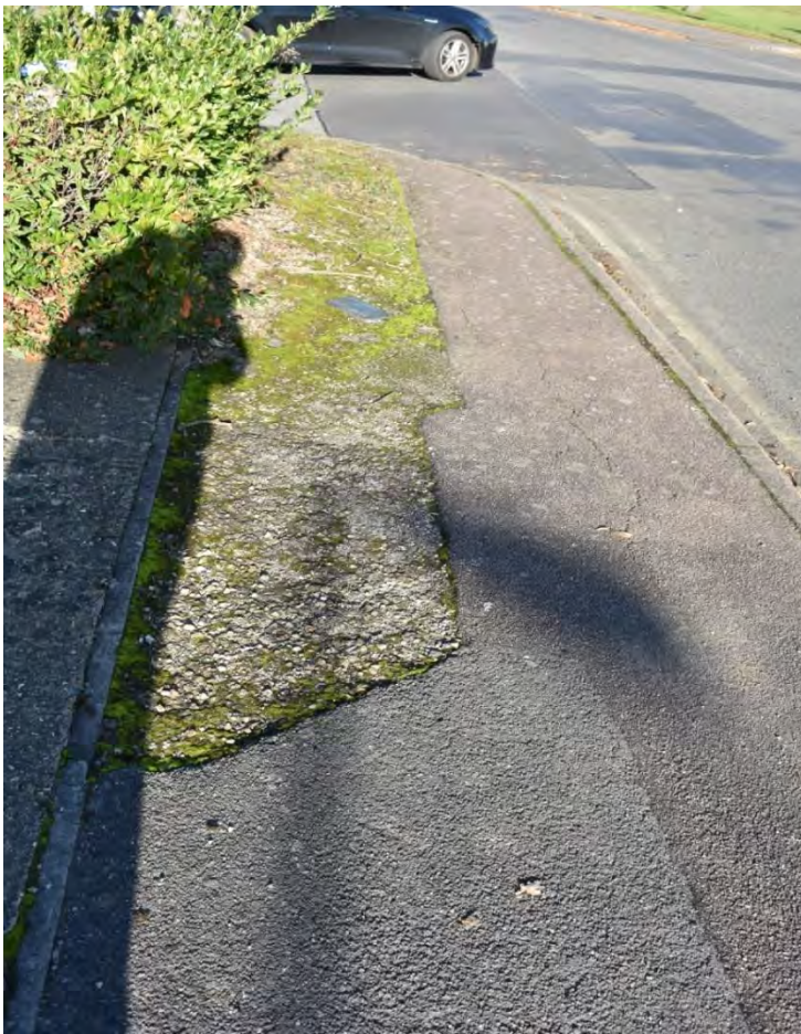
Pavement near Homebase.
